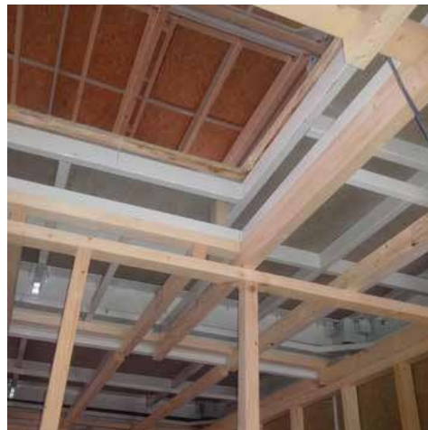
Space between modules
